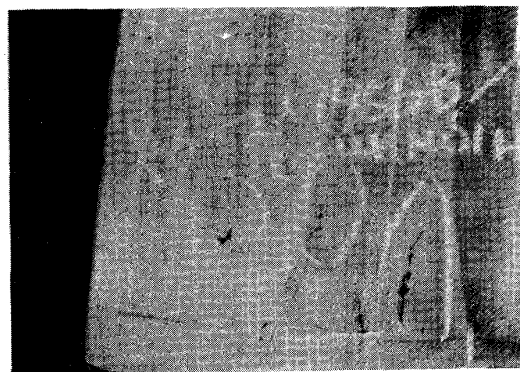
Photo. 1. Cracks on the slab surface after grinding.
