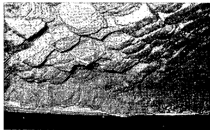
Photo. 1. Old-type roof showing severe spalling. (after 63 heats.)
